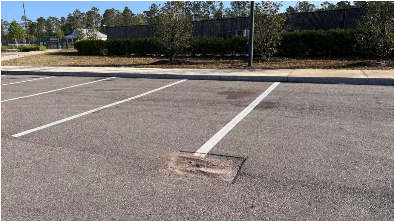
Hole in parking lot at Amenity Center Tennis Courts
