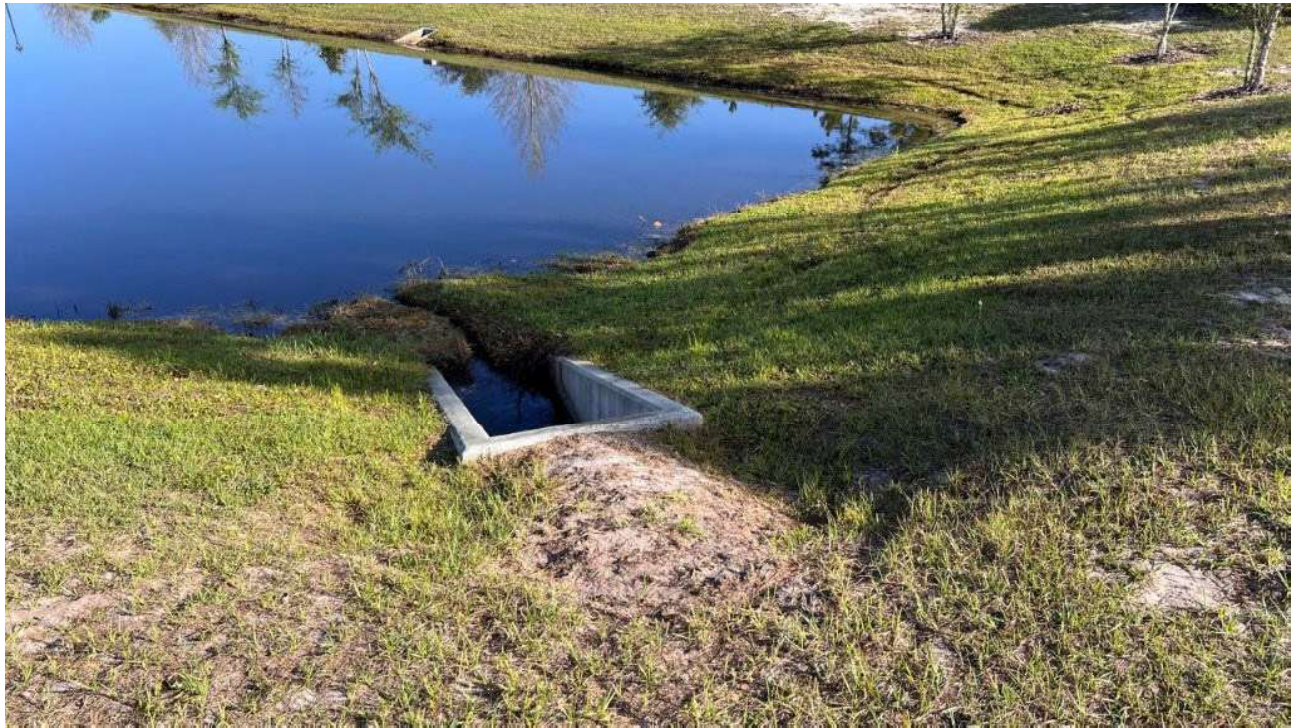
MES erosion located in SMF 203 (Pond 5)
