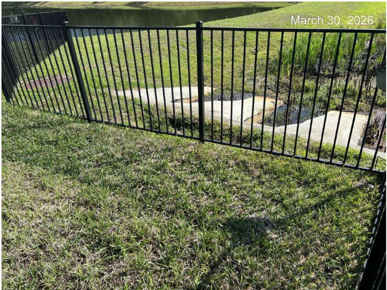
Soil settled at 2290 Oak Stream Drive
