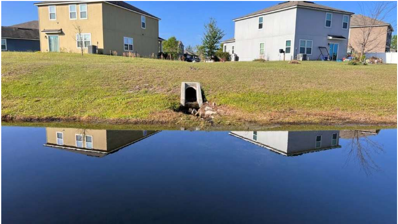
Mitered End Section (MES) erosion located in Stormwater Management Facility (SMF) 203 (Pond 5)
