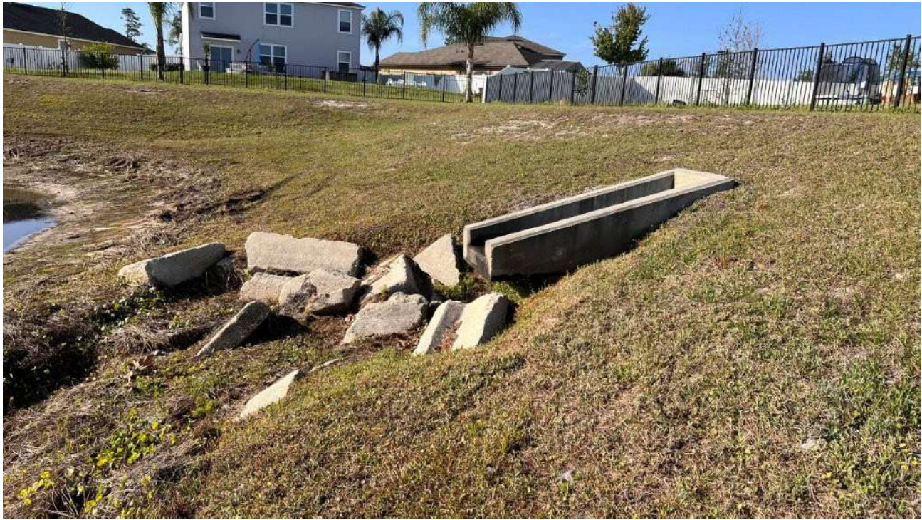
MES erosion located in SMF 204 (Pond 6)
