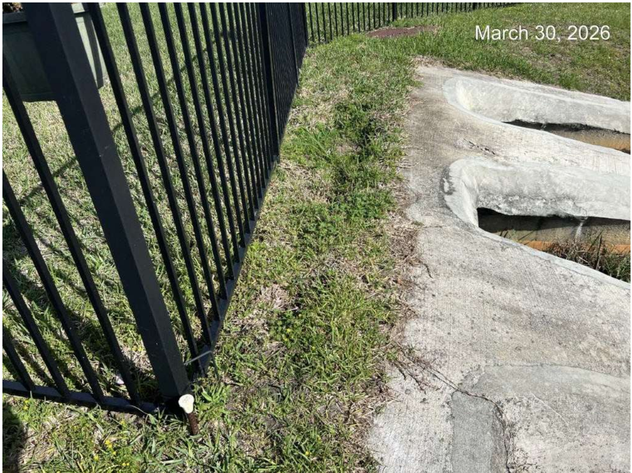
Soil settled at 2290 Oak Stream Drive
