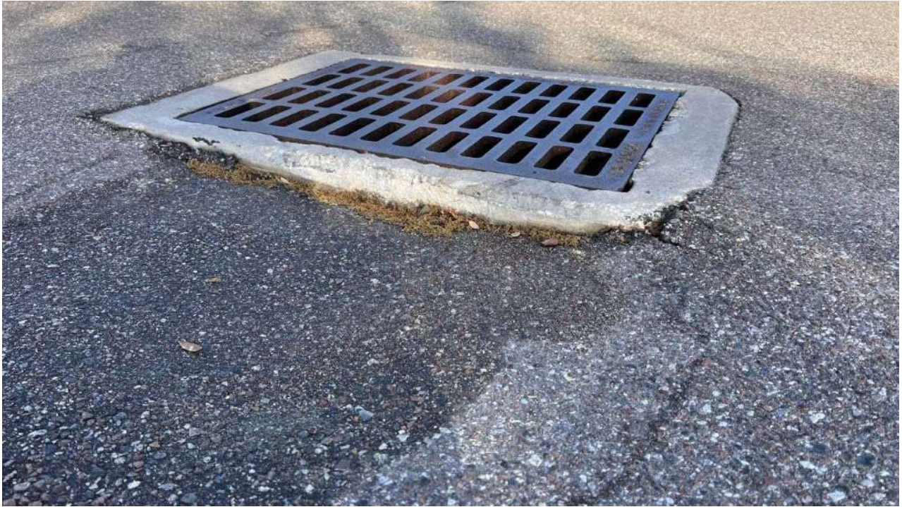
Settling occurring at the inlet - entrance to the Amenity Center
