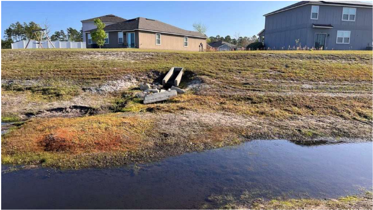
MES erosion located in SMF 204 (Pond 6)
